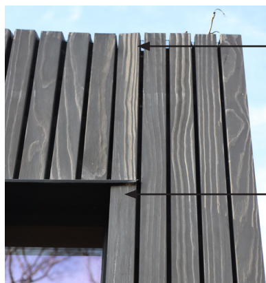
Cupping: more moisture cycling + UV exposure at the top exposed edges
